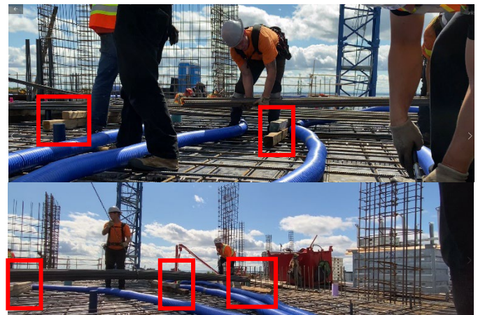
Figure 6 : Double the wooden supports when the reinforcements are placed on the FLIXS networks.
